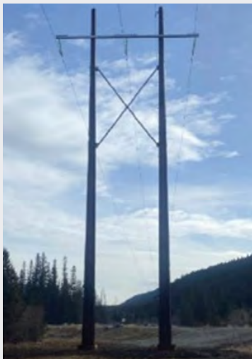
Above: H-frame structure
